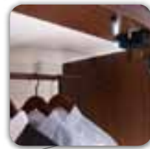
Wardrobe lighting with contact switch
