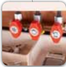
Central gas distributor in kitchen area
